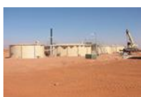
Containerised sewage plant
